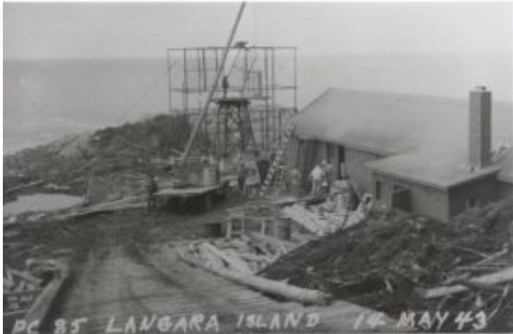
The Operations room adjacent to the Radar transmitter
